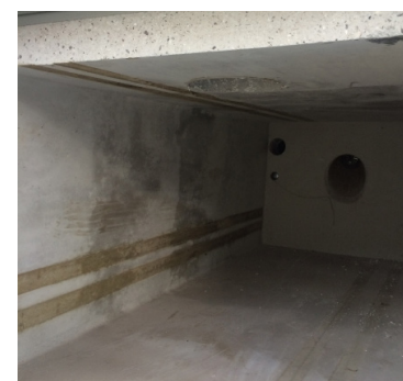
Internal Chamber View
