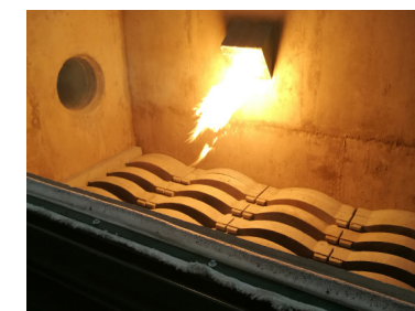
Internal View Burners On
